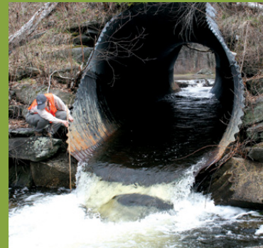
Road crossings with an outlet drop create a barrier in the stream that blocks fish passage.
