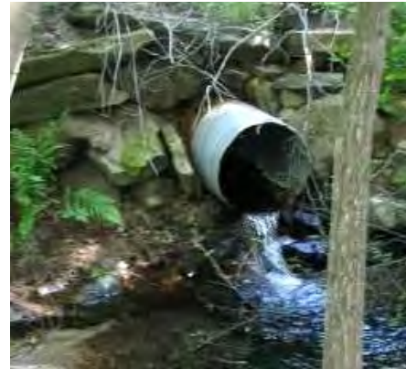
A “perched” culvert on River Road in Windsor, preventing fish passage and resulting in scour at the outlet.
